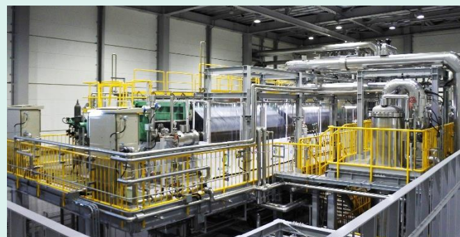
10 MW alkaline water electrolysis system
