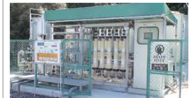
Independent drinking water supply system
