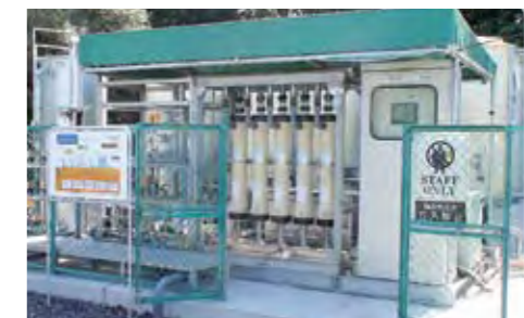
Independent drinking water supply system in Moriyama
