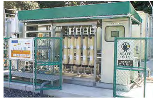
Independent drinking water supply system in Moriyama, Shiga Prefecture
