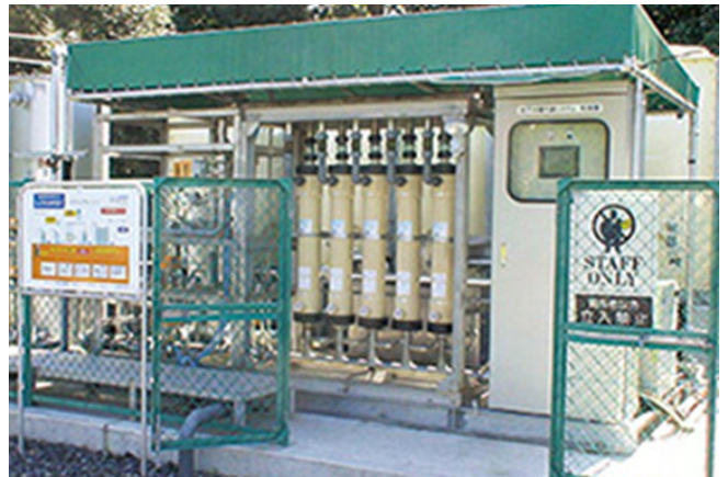
Independent drinking water supply system in Moriyama, Shiga Prefecture
