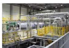
10MW-class alkaline water electrolysis plant
